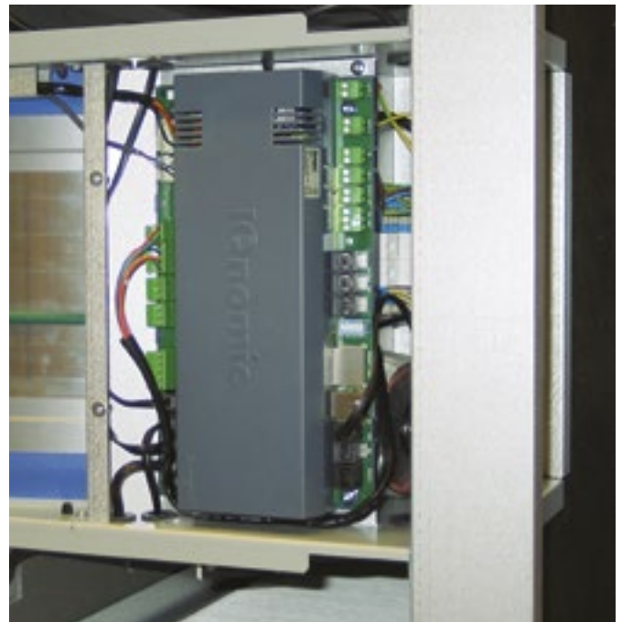
IQnomic control unit.
